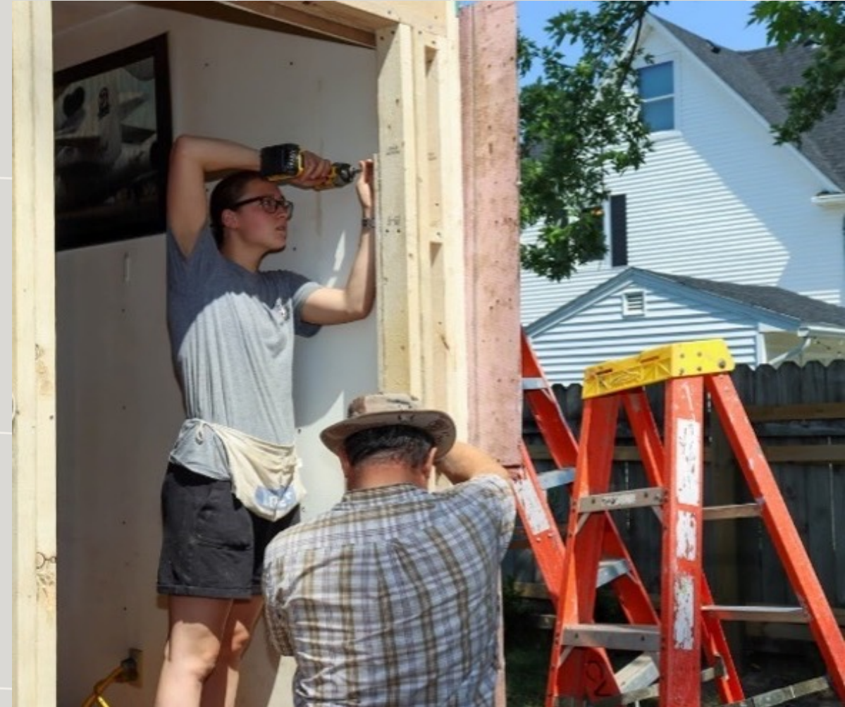
House repair after the 2020 Iowa Derecho. Photo credit: Habitat for Humanity of Iowa
